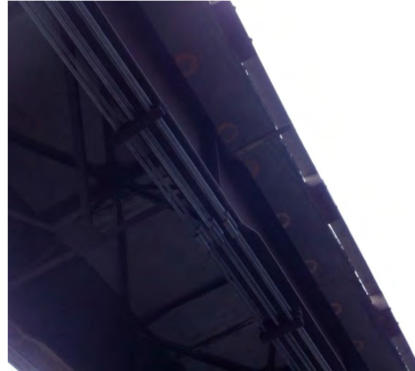
markings under deck panels - for fibre optics hangers?
