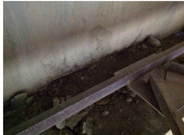
right bank ballast wall damage - rebar exposed
