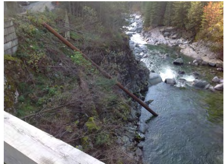
pipe in water on downstream side of bridge
